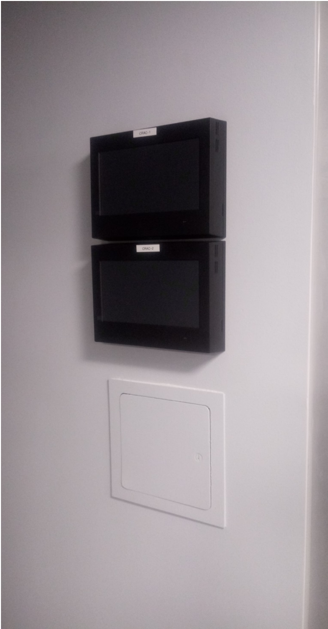
Server Room 122 – CRAC-1 & CRAC-2 Controllers
